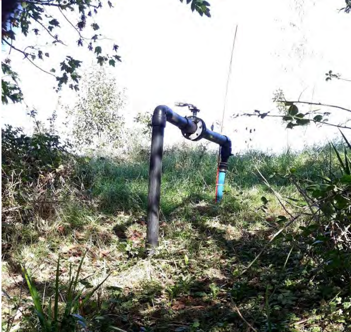
Photo 7 – Gas/leachate infrastructure observed in the side slope of the Windmill Quarry authorised landfill. It is unclear if this infrastructure is active.
